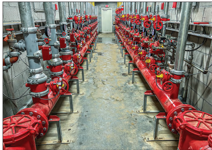
Screening and conveyor deluge valves
