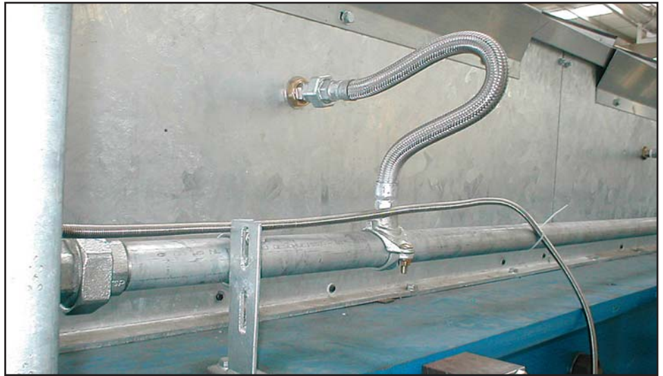
Lower heat tunnel fine spray nozzle.
